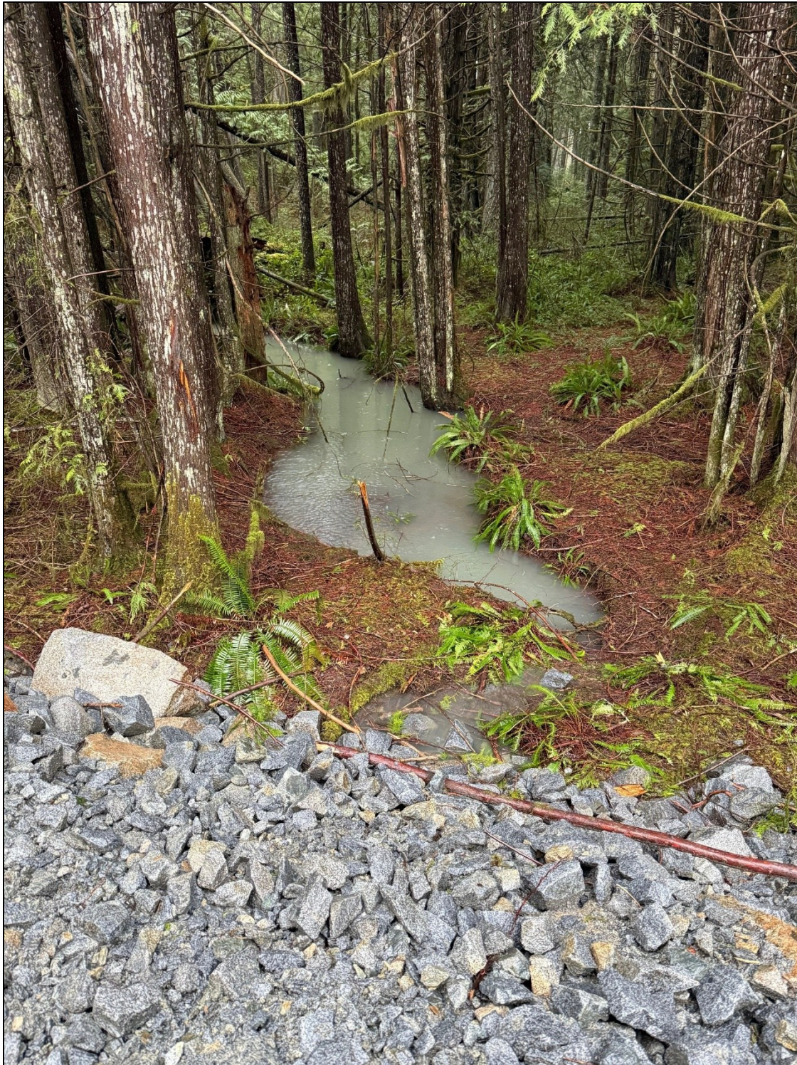
Photo 3: Visible sedimentation entering Blackwater Creek from road runoff during construction.
